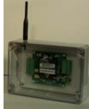
Base Station mounted at PACS panel
